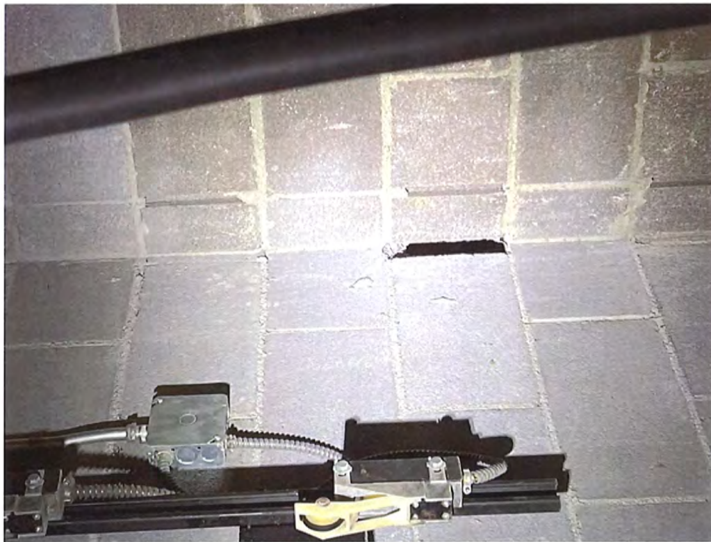
Hole to be filled in elevator shaft
