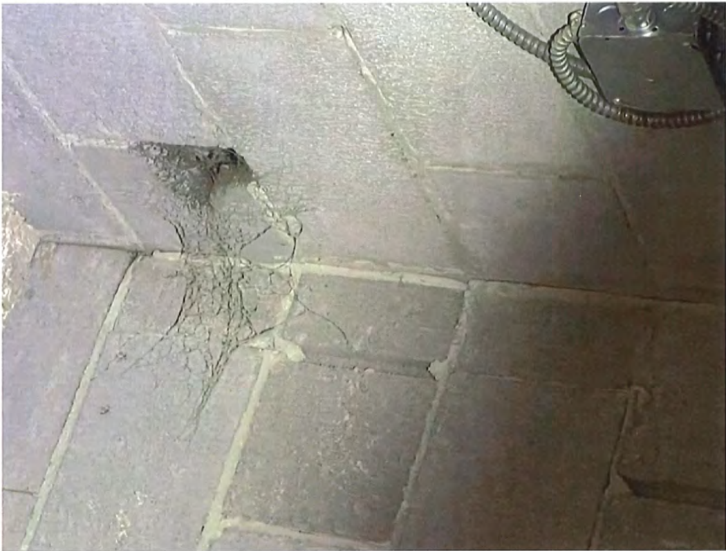
Hole to be filled in elevator shaft
