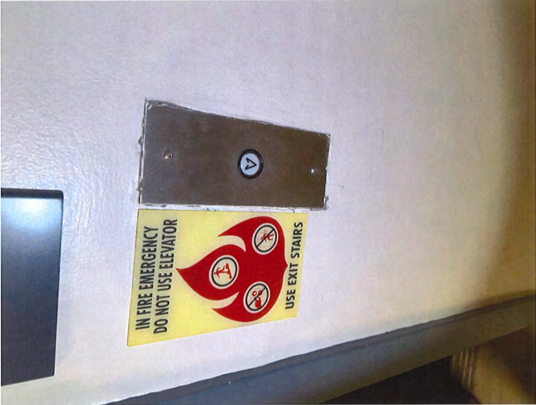
Plate at exterior of elevator
