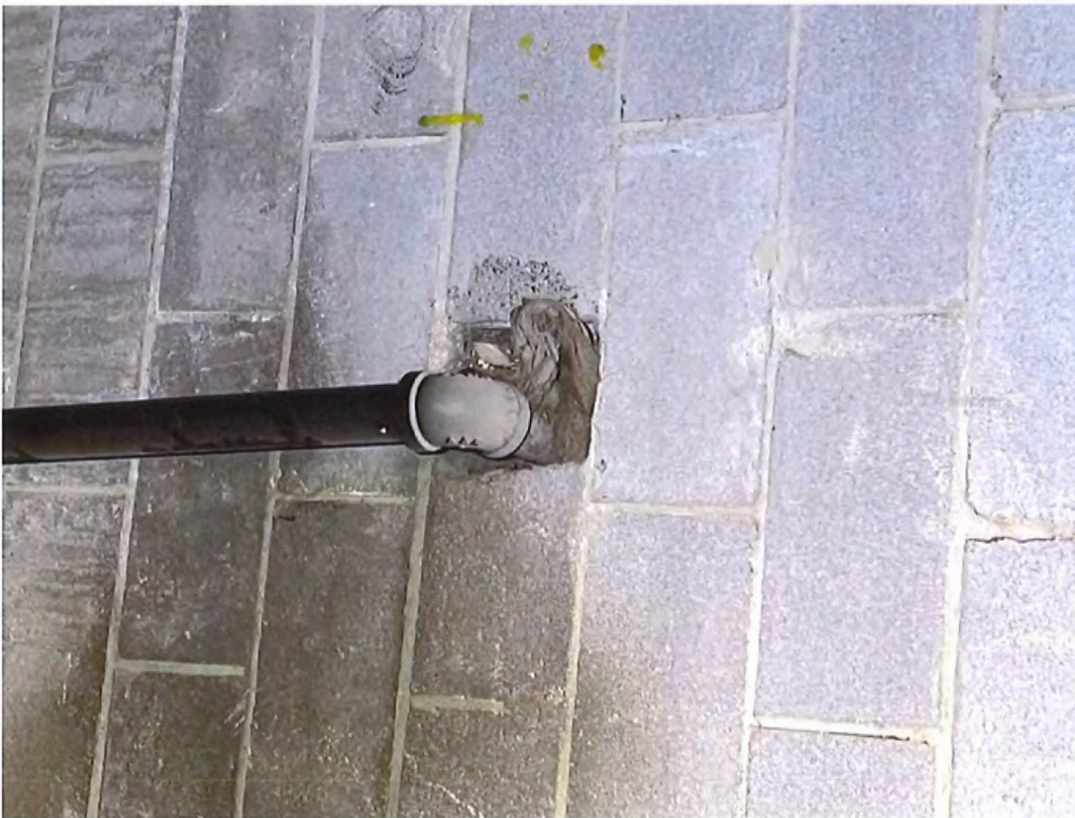
Hole to be filled in elevator shaft
