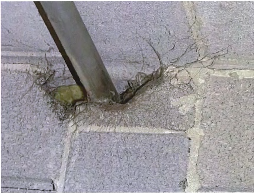
Hole to be filled in elevator shaft
