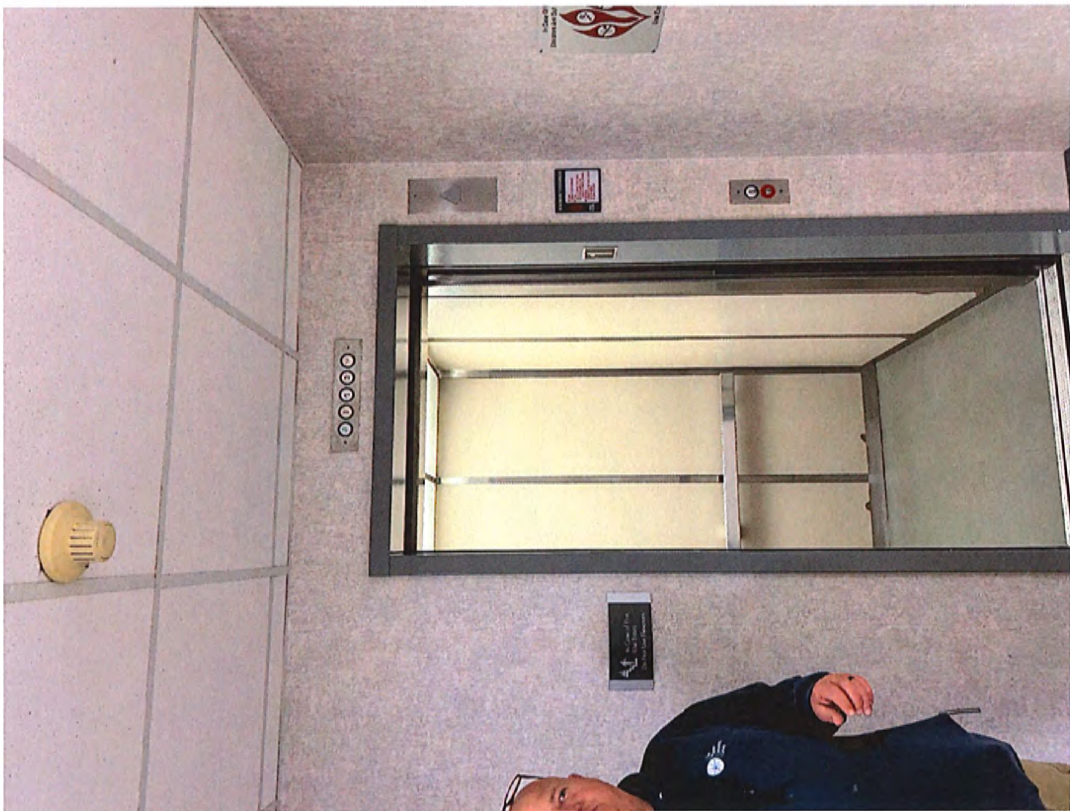
Plates at elevator
