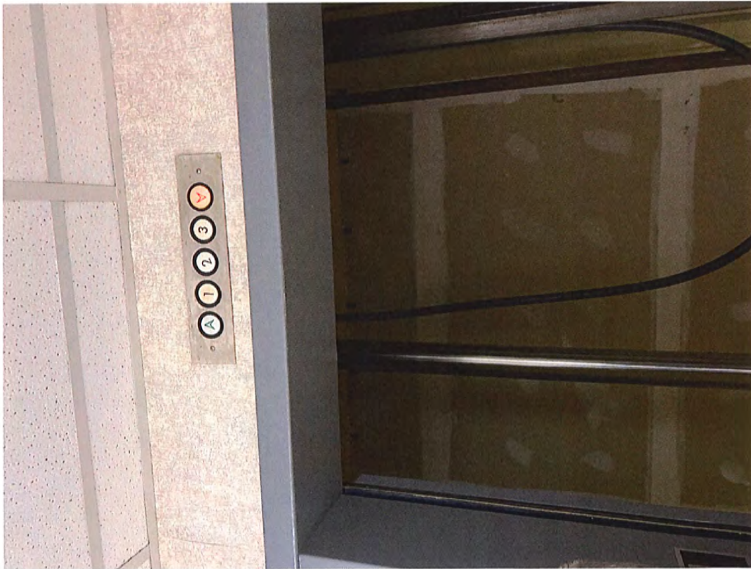
Plates at elevator
