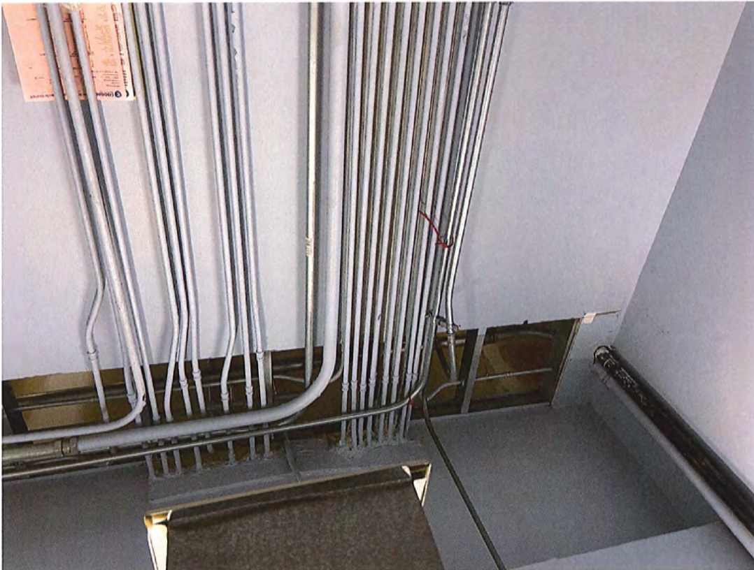
Wall between elevator machine room and electrical room. Room to be fire rated and extend wall to top of deck.
