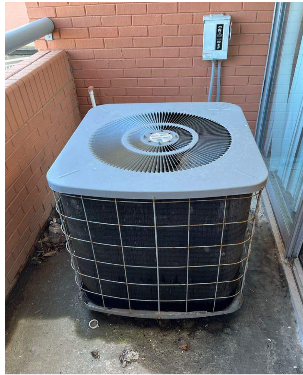
3 BUILDING 900 BALCONY OUTDOOR UNITS SCALE: NTS
